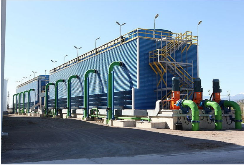
Fig. 1.1. Industrial cooling towers in a power plant.
