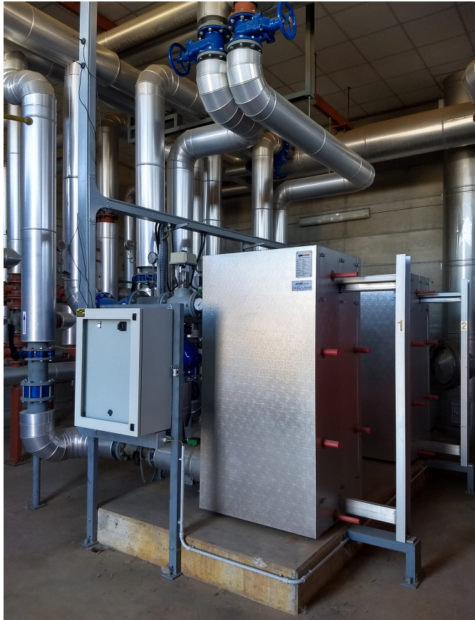
FIGURE 2.16: District heating substation. The plate heat exchanger is placed inside the silver box with red exiting rods.
