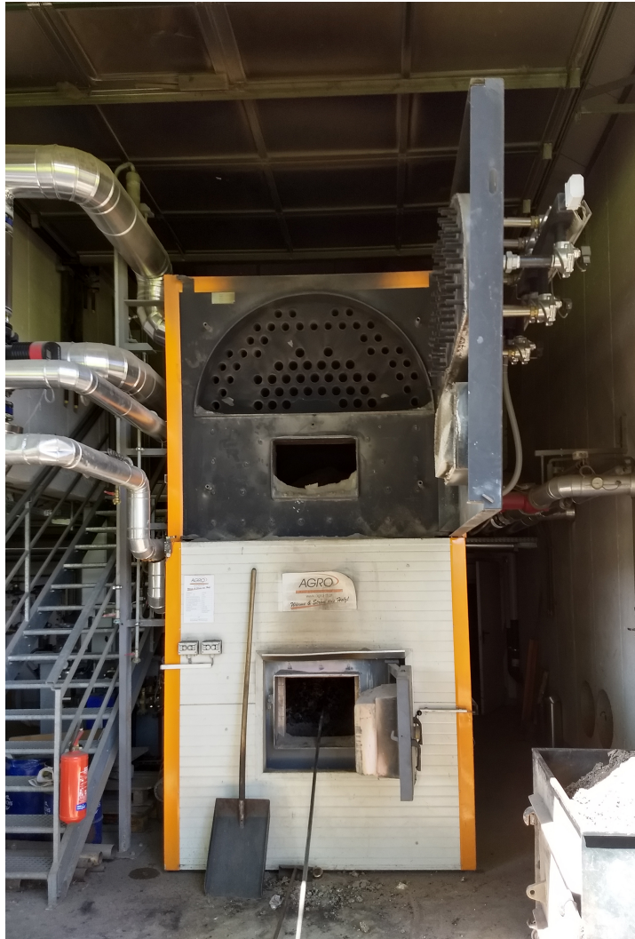
FIGURE 2.15: District heating biomass boiler, thermal power of 800 kW. Here shown during summer period maintenance.
