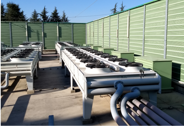
FIGURE 2.1: Industrial dry coolers.
