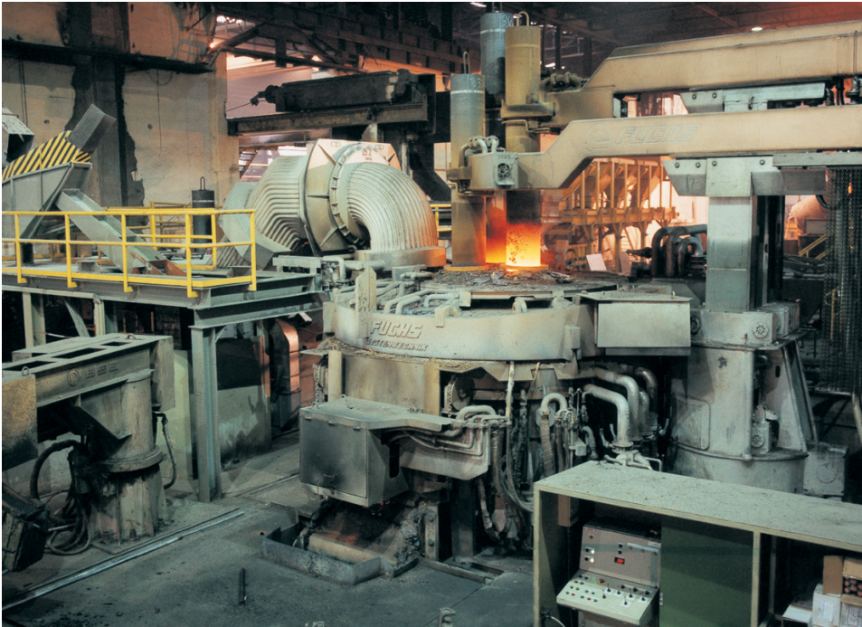
FIGURE 4.2: An electric arc furnace, note the elbow with a gap collecting the hot flue gases exiting the furnace (left side of the electrodes) source: https://ru.wikipedia.org/wiki .
