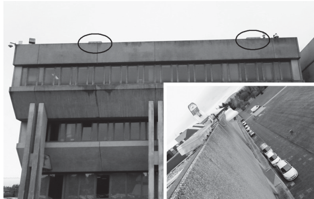
Figure 6.3: The prototype installed on the roof of the University building. The two arrays are encircled.
