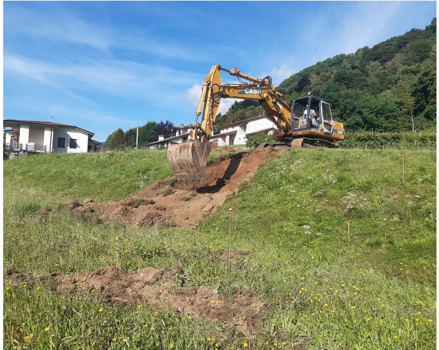
Fig. 8 - The fault scarp near Miane (Fig. 5 for location) during the trench excavation.
