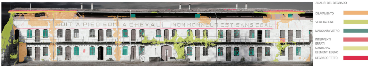
Fig. 2 The façade of the Napoleonic barrack (students: Andreottola, M., Bonadimani, A., Masutti, A., Roman, O., and Tudor, D.).
