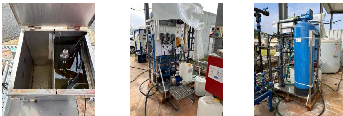
Figure 1 AOP Pilot plant equipped with on-line sensors.
