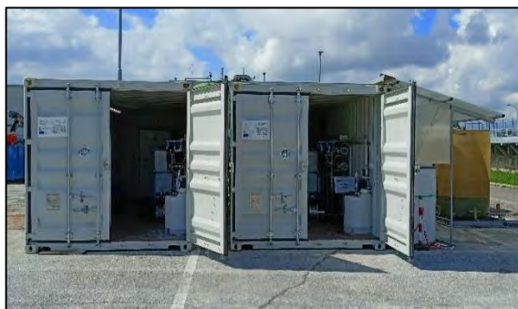
Figure 2 – NF/RO Pilot Plant
