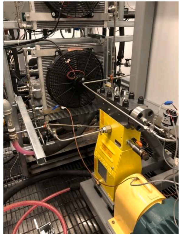
Fig. 2. Photo of the pump installed in the CO 2 test stand.
