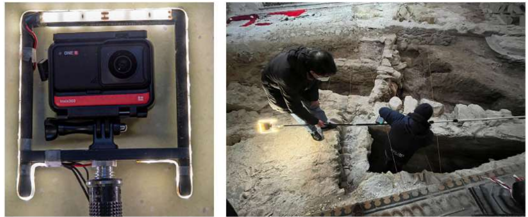
Figure 1. Details of the prototype for the 360° borescope and the on-site work with the system installed on a telescopic pole.
