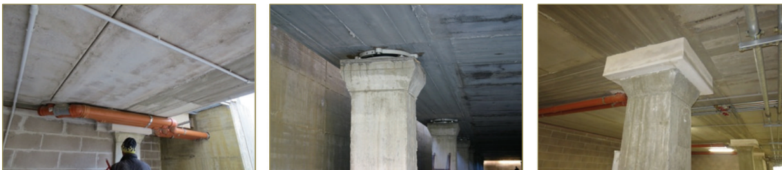
FIGURE 17: Images of waste water pipes at an interface area between the mobile and fixed portions of the building and two columns before and after the installation of the fire-protection plasterboard on the isolators.
