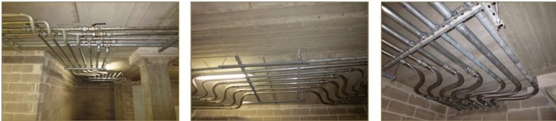
FIGURE 16: Images of gas pipes at an interface area between the mobile and fixed portions of the building.
