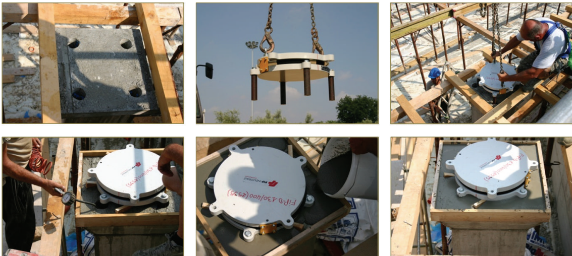
FIGURE 14: Images of the installation works of a DFP isolator over a column.
