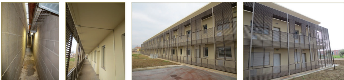
FIGURE 18: Images of a wing of the perimeter interspace between the retaining wall of the basement and the building, the thermal expansion joint between B2 and B3 blocks, and the main façades of B1–B3 and B4 blocks.
