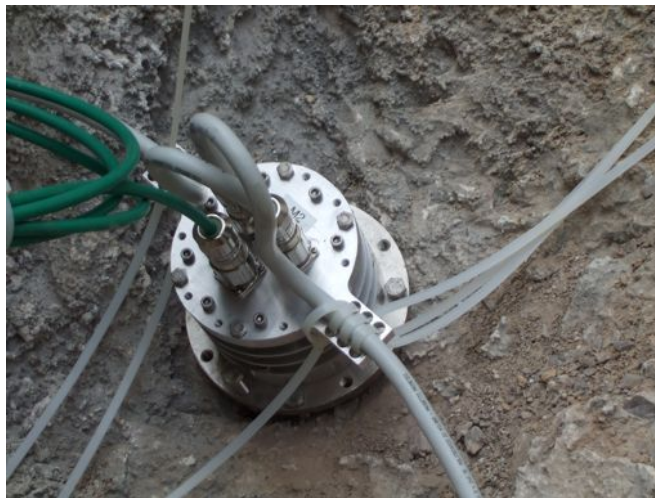
Figure 2.1: Sensor used for the vibration monitoring.
