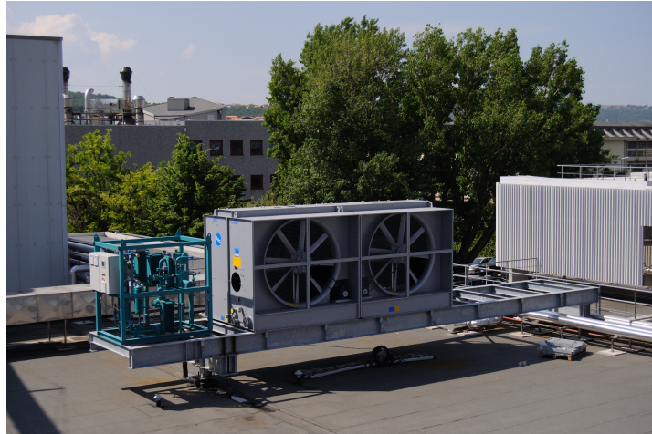
Figure 6.4: Heat recovery plant view
