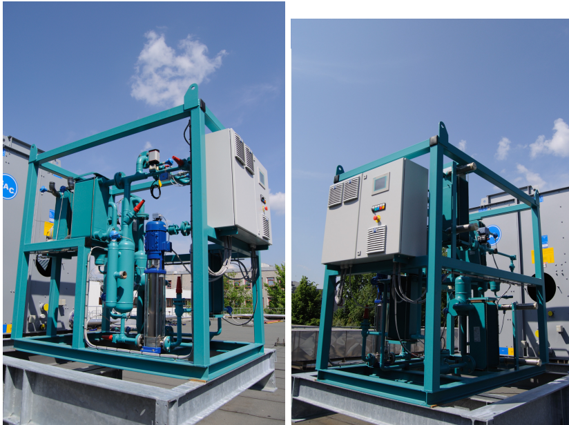
Figure 5.15: Two views of the absorption chiller prototype as installed
