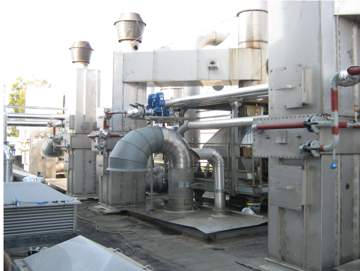
Figure 6.2: Heat recovery plant
