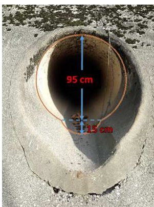
Figure 3.12: Some pictures about the survey of the sewers, a fundamental step in order to model the sewer and hydraulics of runoff and the end-of-pipe section
