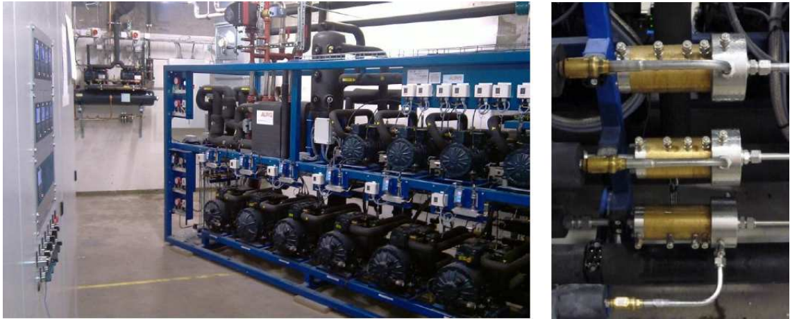
Fig. 3.26 – Left-hand side: 2 parallel compressors, 4 HS and 4 LS compressors; Right-hand side: 1 liquid ejector at the bottom, 2 vapour ejectors at the top (Hafner et al., 2014c).
