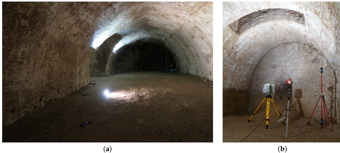
Figure 2. (a) A section of the tunnel of the Impossible bastion. (b) Setup of the Leica ScanStation C10 over a traverse mark and target pole over the back target.
