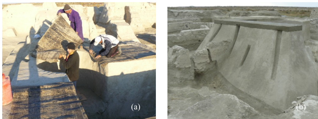
Fig. 5.91. The positioning of tarred paper (a) and the final sacrificed layer (b)
