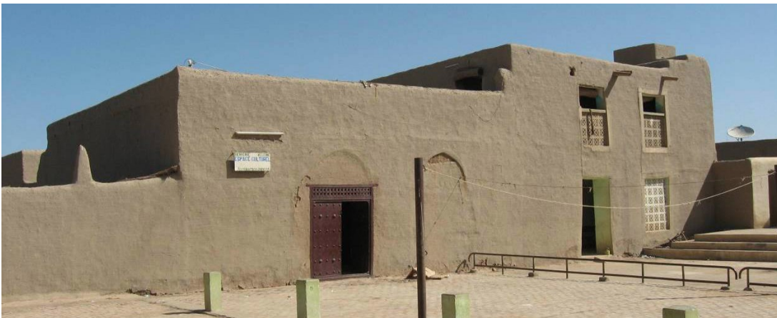
Fig. 4.24. Djenné (Mali), the South façade of the Youth House before the intervention in 2009
