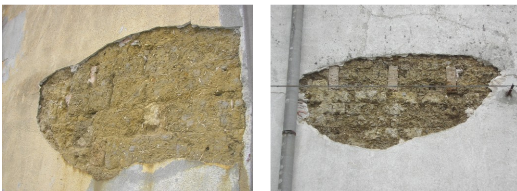
Fig. 5.1. Province of Cagliari in Sardinia (Italy), a sand cement plaster can get separated from the earthen walls because of the vapour pressure and the low cohesion between the two materials
