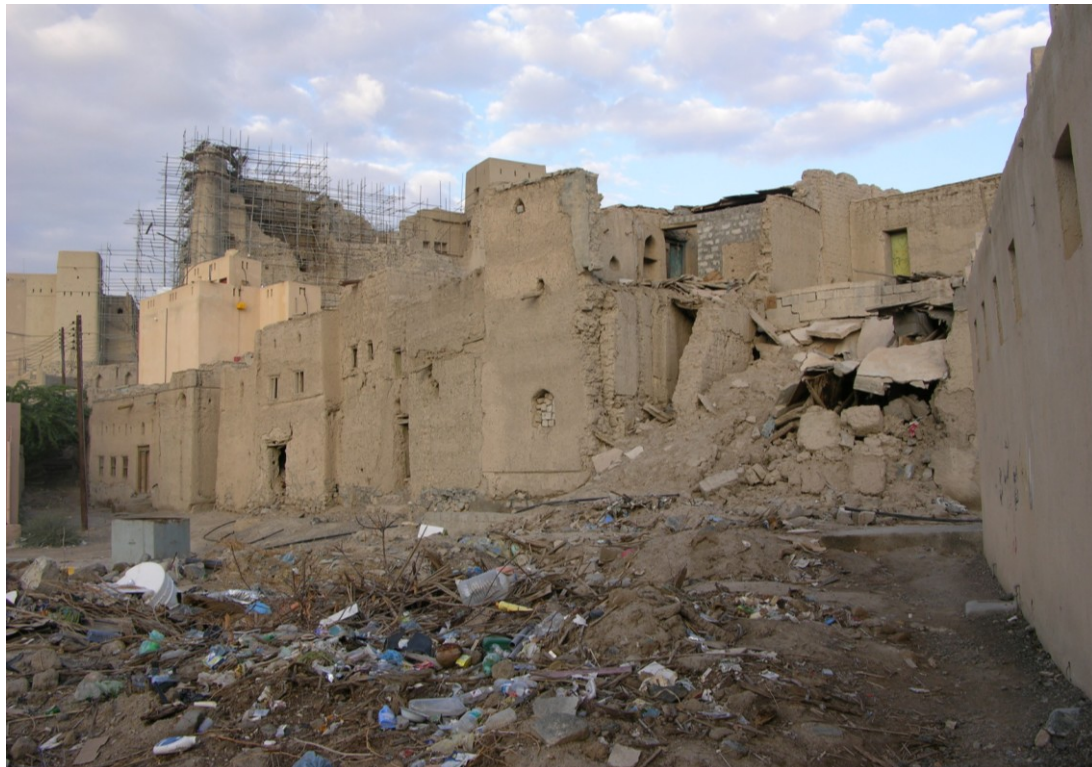
Fig. 5.92. Bahla parking fort (Oman), the area is in a bad state of decay, the rubbish is spread all around and it is not cleaned periodically
