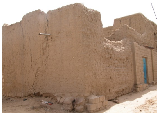
Fig. 5.45. Mali, Djing quarter, cracks along the walls
