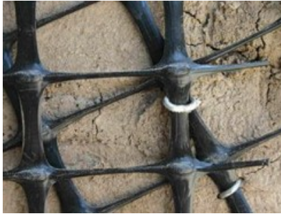
Fig. 5.63. Lima (Peru), type of Geo-grid applied on adobe wall and its fixing system
