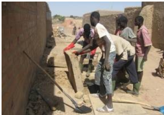
Fig. 4.16. Djenné (Mali), rehabilitation of the canal: cleaning and improvement of drainage system
