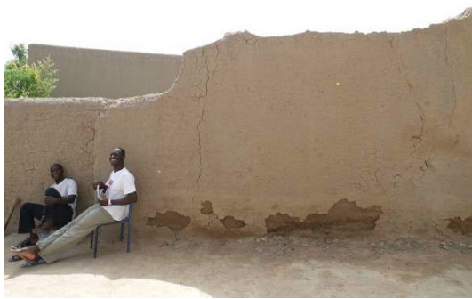
Fig. 5.17. Djenné (Mali) the Youth House: the basal erosion of the wall due to the dissolvable salts
