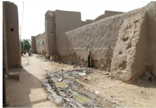
Fig. 5.18. Djenné (Mali) the Youth House walls in Sankoré road: the basal erosion of the wall due to the dissolvable salts
