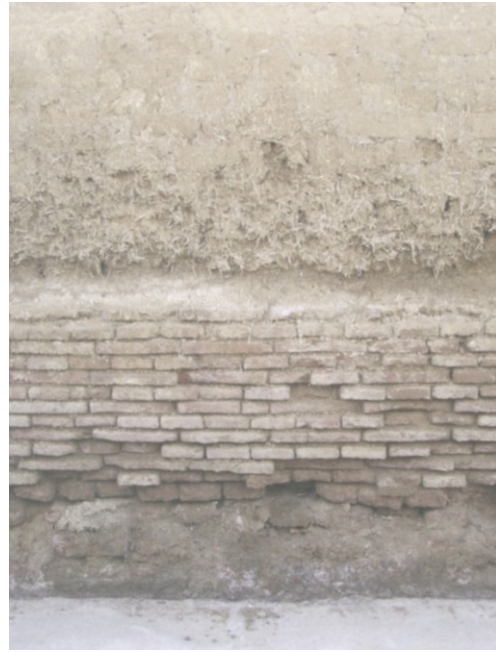
Fig. 5.15. The splashing effect of the rain along the joint wall-basement, already damaged by the capillarity
