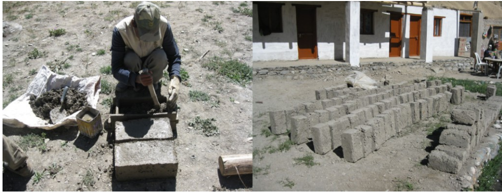
Fig.4. Studying the vernacular building technologies: production of the the pakbu , the local mud brick (credits: Désirée De Antoni)
