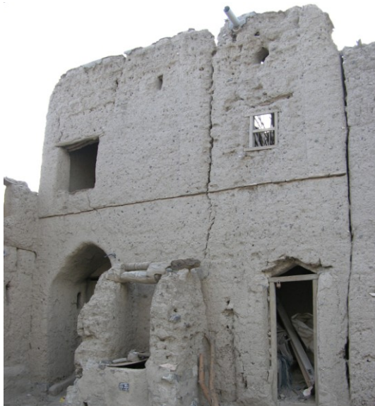
Fig. 5.42. Bahla (Oman), Harah quarter, cracks along the walls
