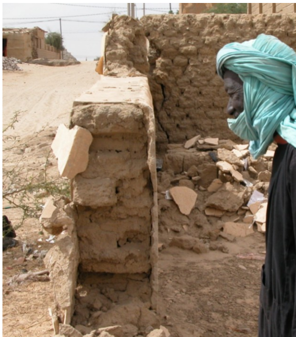
Fig. 5.74. Timbuktu (Mali), cement plaster does not allow the wall breathe, causing the stagnation of the water infiltration and the collapse of the structure
