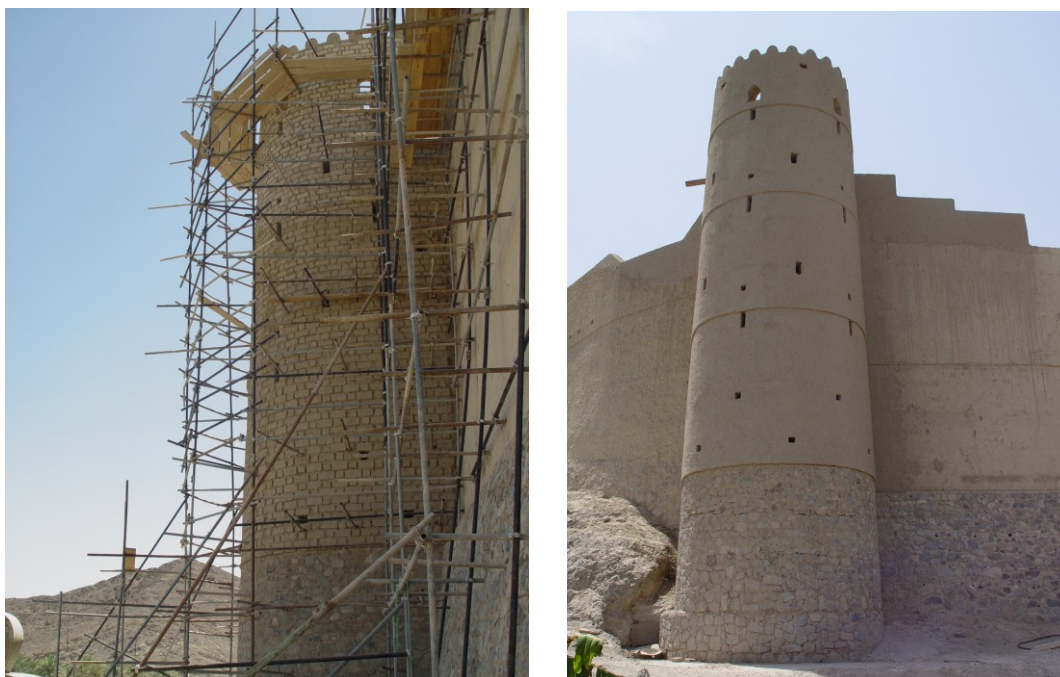
Fig. 5.51. Bahla (Oman), North West Tower of the Fort under reconstruction and after the intervention
