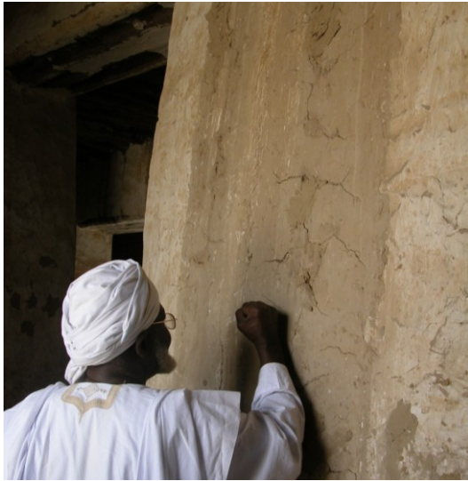
Fig. 5.20. Mali, the water infiltrations through out the roof
