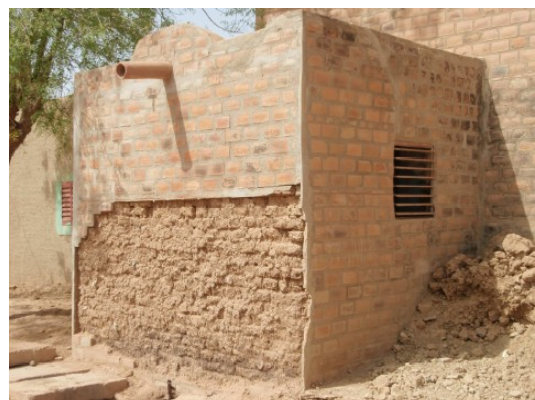
Fig. 4.43. Djenné (Mali), the damages of an earthen masonry, plastered with terracotta bricks
