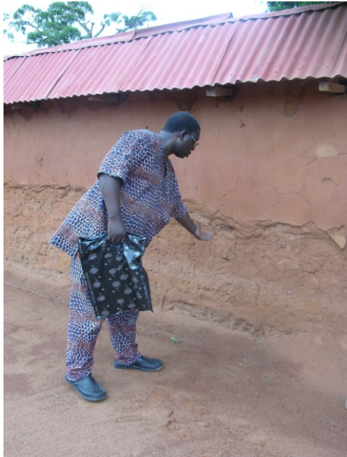
Fig. 5.14. Abomey (Benin), the basal erosion of the wall due to the direct action of the rain as well as the capillarity
