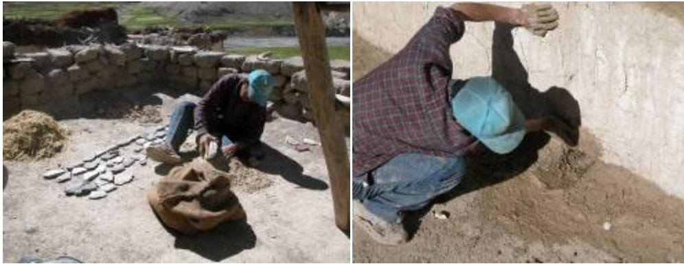
Fig.10-11. Creation of the improved joint using markallak mixture and finely chopped straw with stone joint cover.
