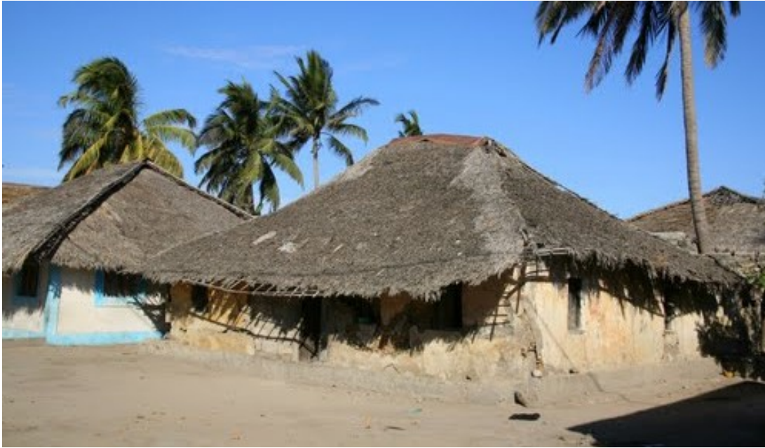
Fig. 3.5. Macuti Town (Mozambique), the earthen houses are made with the wattle and daub technology while the roof is covered with palm leaves
