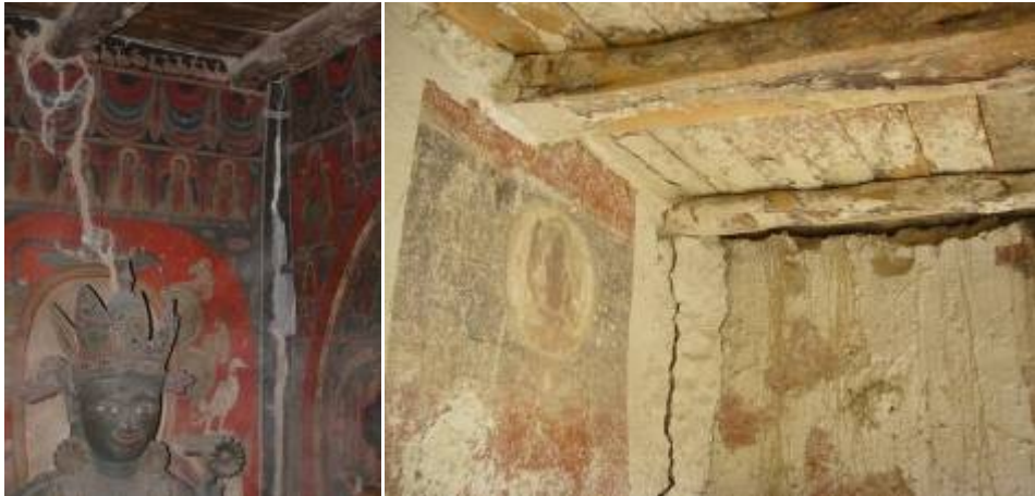
Fig.2-3. Degrading action on the earthen wall decorations caused by infiltrations of water inside the temple.
