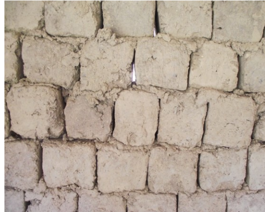
Fig. 5.2. Kanji, Ladakh (North India), the lack of earthen mortar along the vertical joints
