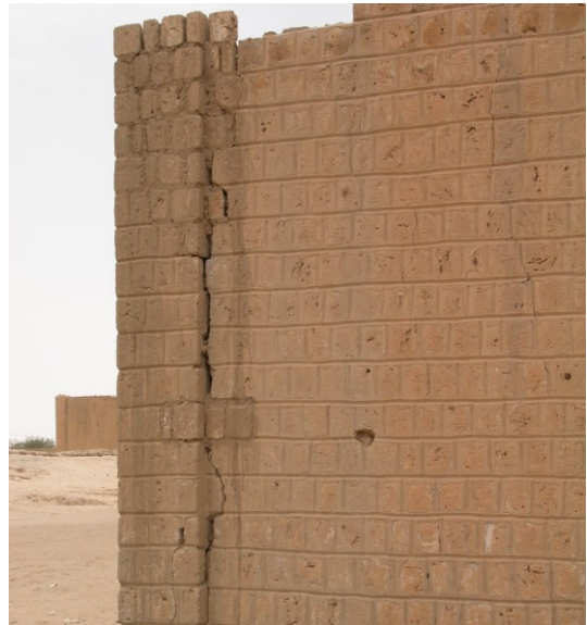
Fig. 5.43. Sankoré (Mali), a big crack at the wall corner
