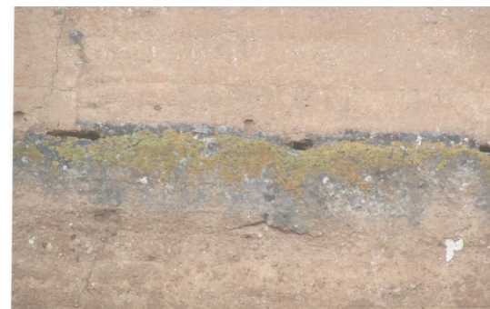
Fig. 5.23. A rammed earth wall affected by parasites like moss
