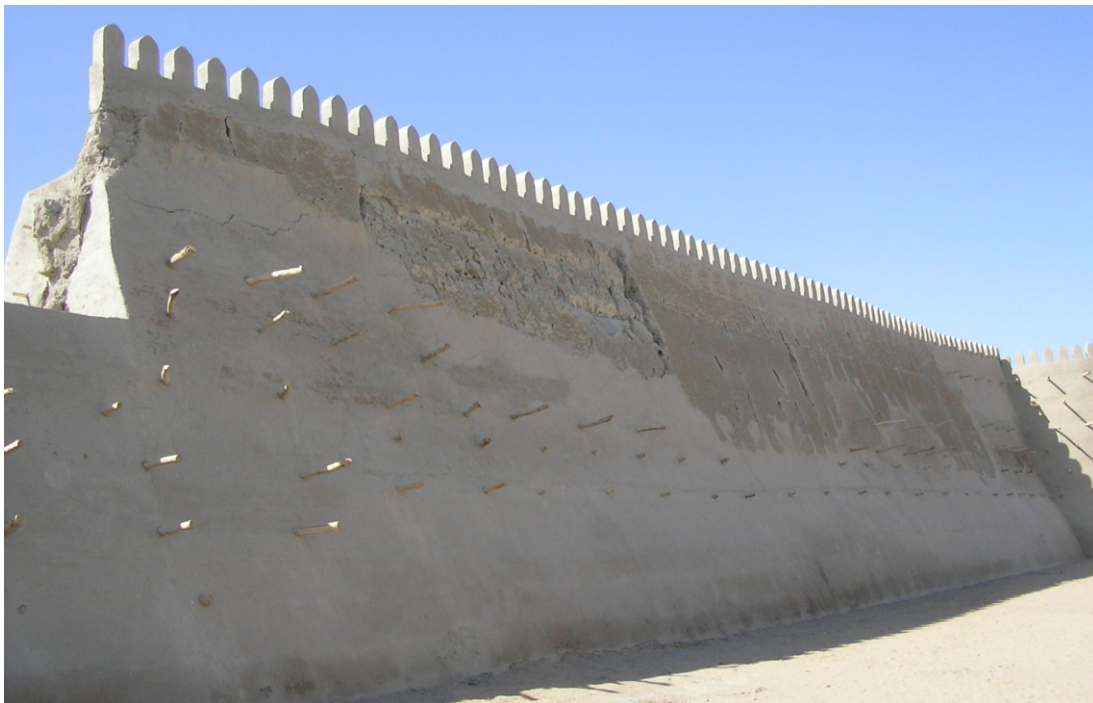
Fig. 5.19. Bukhara (Uzbekistan), the swelling and the loss of the earthen plaster which is subjected to harsh winter and hot summers
