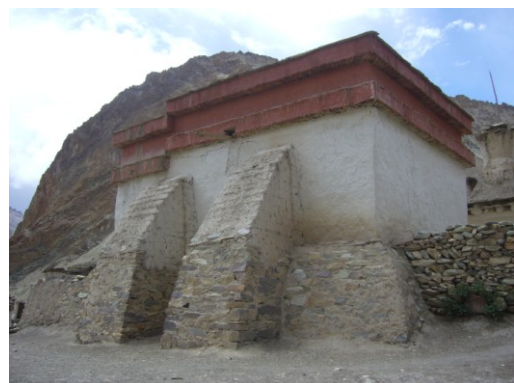
Fig. 5.69. Kanji, Ladakh (North India), two earth/stone buttresses avoid the overturning of a load-bearing wall in a private temple
