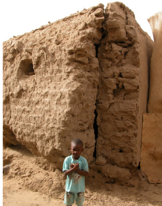
Fig. 5.13. Timbuktu (Mali), decay of an earthen house due to the direct action of the rain and the stagnation of the water at the basement
