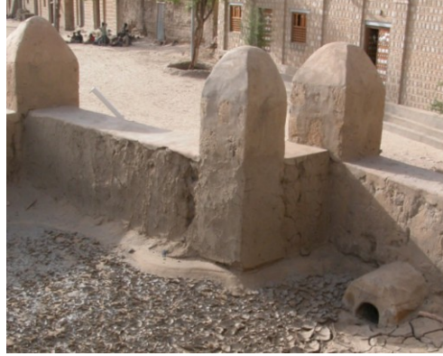
Fig. 5.11. Sankoré (Mali), the erosion of the mosque roof after the water stagnation
