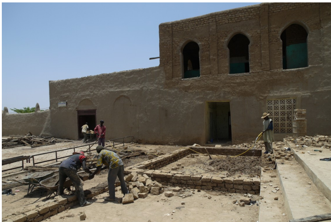
Fig. 4.32. Djenné (Mali), the rehabilitation of the Youth House of Djenné: the South facade aspect in 2011
