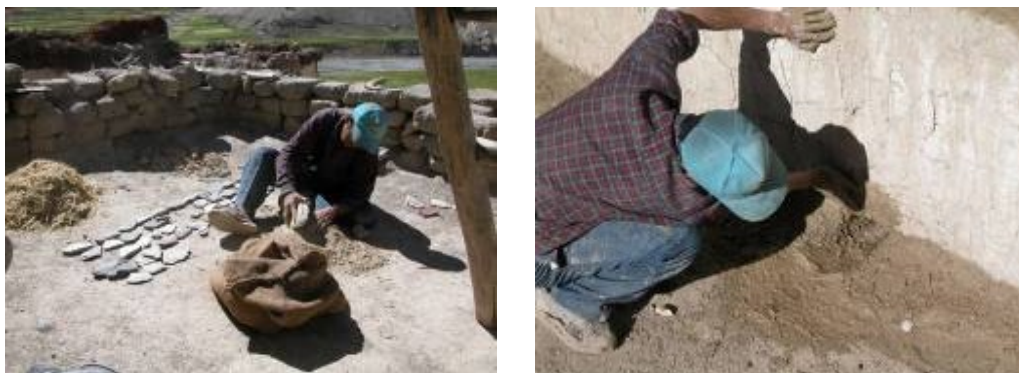
Fig. 5.88. Kanji, Ladakh (North India), creating improved joints, using earthen mixture and finely chopped straw with stone joint cover
