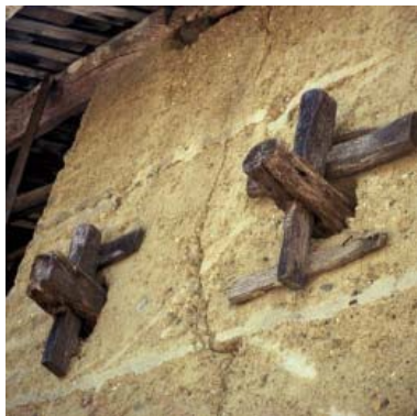
Fig. 5.67. Transversal wooden ties
