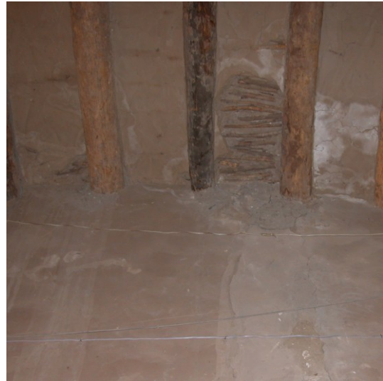
Fig. 5.21. Timbuktu (Mali), the roof degradation due to rain and wind
