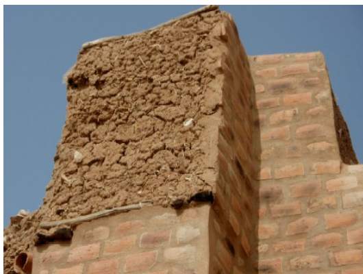
Fig. 4.42. Djenné (Mali), the damages of an earthen masonry, plastered with terracotta bricks
