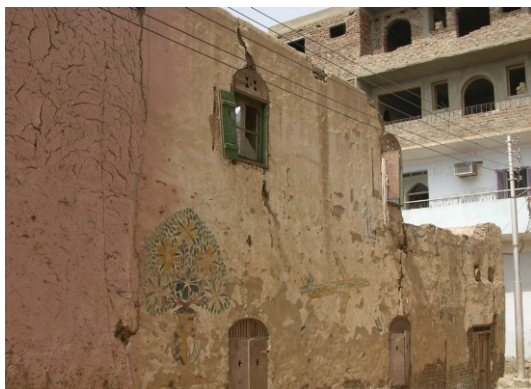
Fig. 5.44. New Gourna (Egypt), cracks along the walls and at the openings
