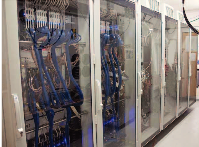
(a) Photo of the new electronic room
