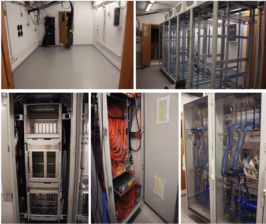
Figure 4.20: A temporal sequence of the renovation of the electronic room. (Images credit: J. L. Lemus)
