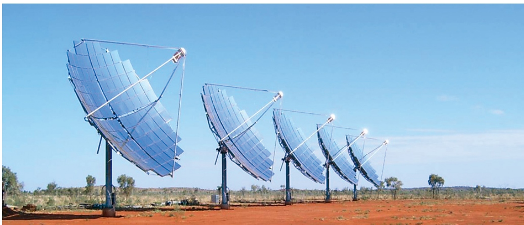
Figure 3.12: Solar dish array (by Solar System Ltd)
