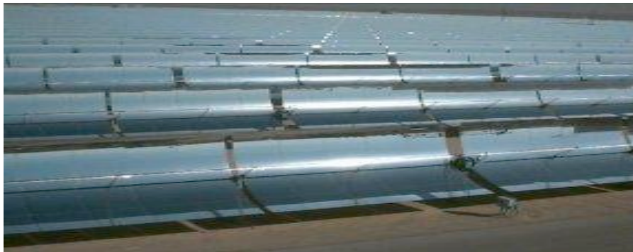
Figure 3.3: Parabolic trough power plant.
