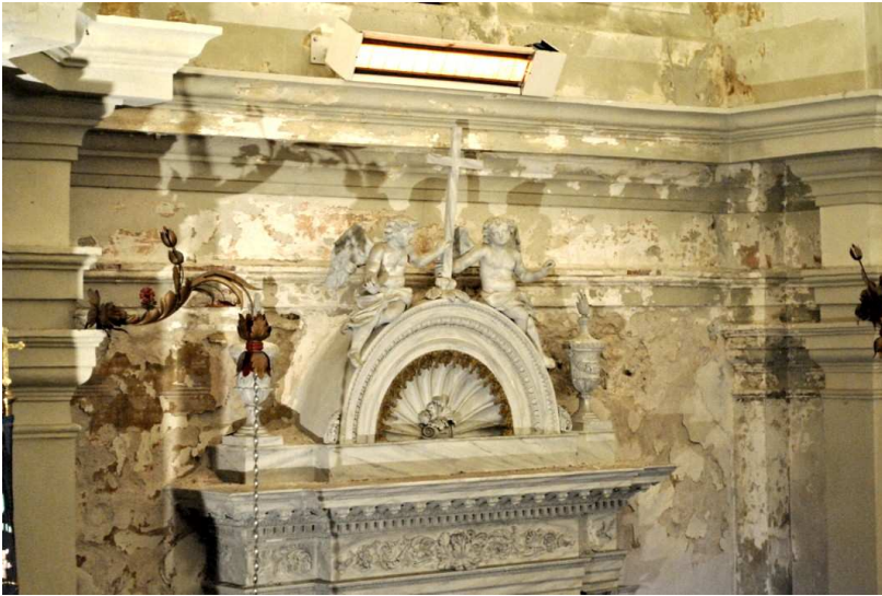
Figure 1.5: Detail of an internal coating detachment of the parish church of Nogaredo di Prato (UD). The damage could be caused by a combined effect of rising damp, rain infiltration and superficial condensation also due to the heating system.
