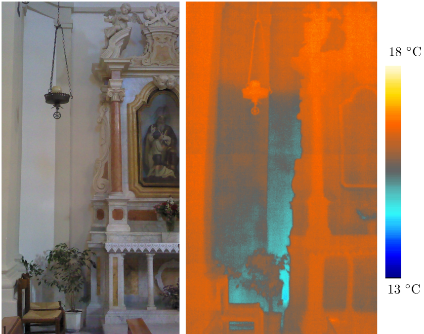
Figure 1.6: Detail of the internal side of the restored wall of the parish church of Raspano (UD). After the restoration the rising damp is not visible but the evaporative moisture transfer at the surface could be visualised with infrared photography. The hygroscopic coating allows the moisture migration without damage.
