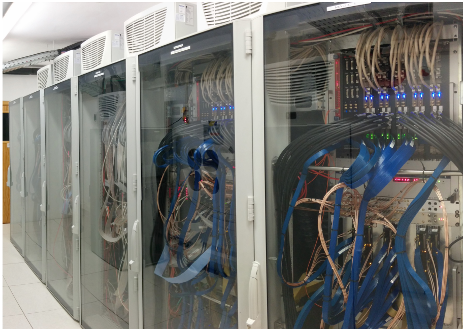
FIGURE 2.6: The electronic room of the MAGIC telescopes where readout and trigger system are hosted. The six racks containing M1 and M2 electronics are visible. In front of them there are also two additional racks containing the Sum Trigger electronics system. From [32].
