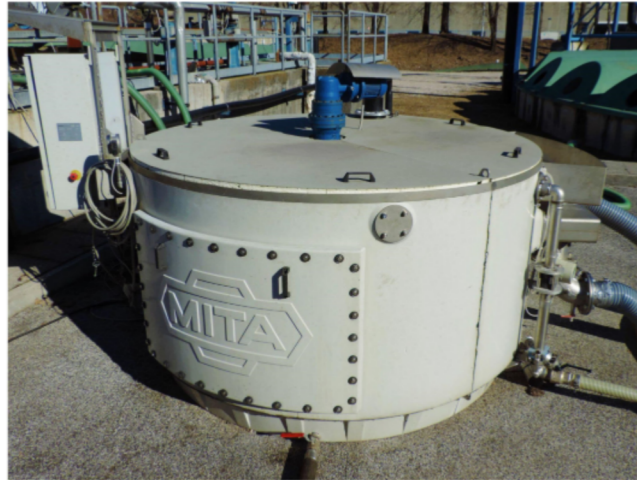
Figure 3. Photograph of the pilot cloth filtration plant installed in the studied wastewater treatment plant.
